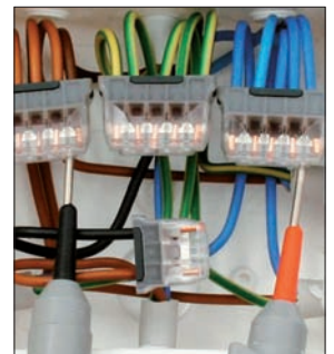
Testing connection by means of the probe whose diameter is 2 mm in the external junction box
